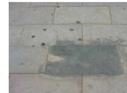
Poor quality reinstatement and chewing gum deposits
