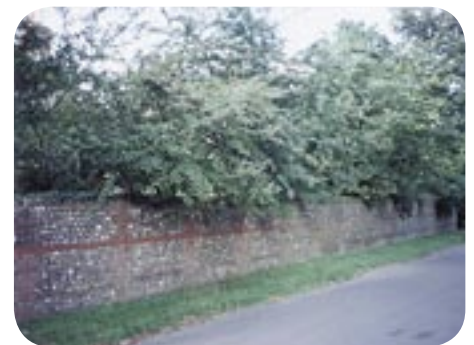
19th century brick and flint boundary wall to The Cottage, Up Street
