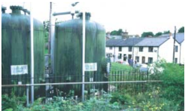
Public utility companies should consider the visual impact of their installations
