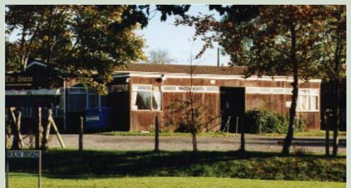
The delapidated Village Hall
