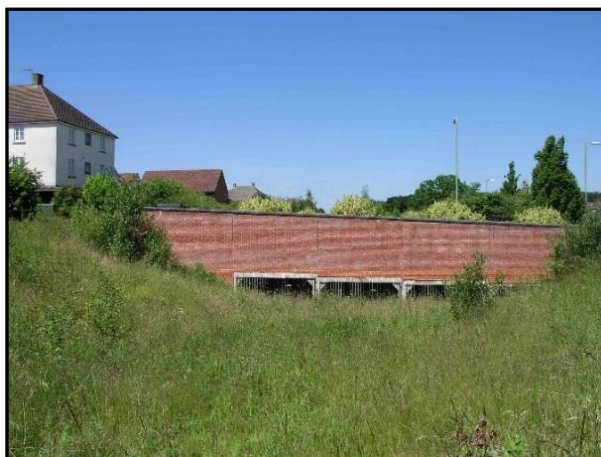
Tunnels under the roads at Marnel Park in Popley allow Great Crested Newts to move through the development
